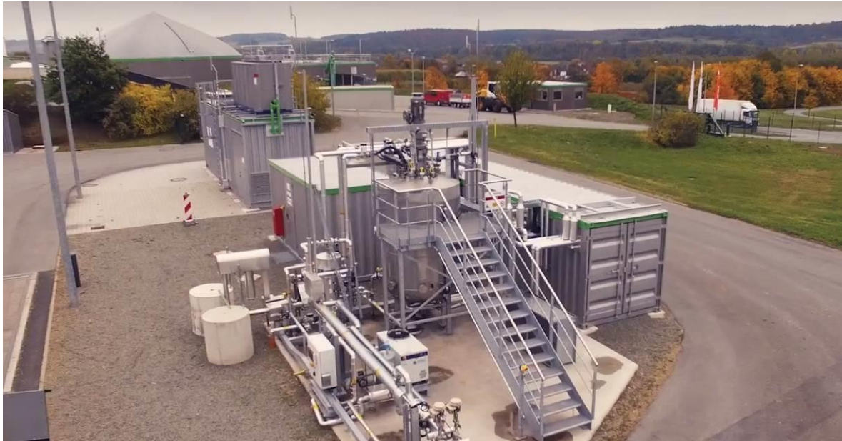
Figure 103 – Installation de Allendorf (300kW, 2015), source Viessmann
